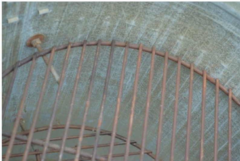
Figure 27.5 Bolts hold up the grate.
